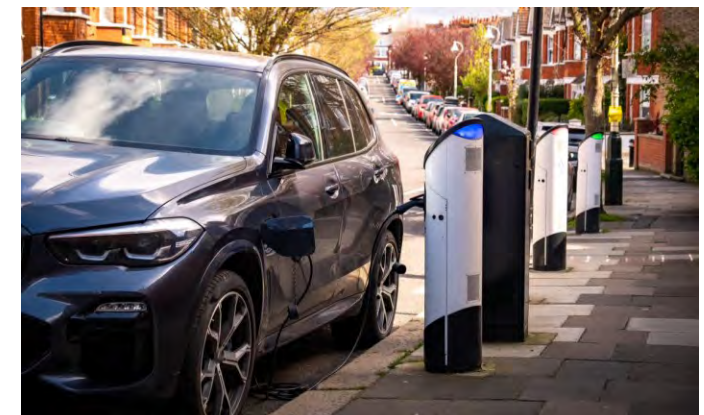
Figure 14 Electric vehicle charge point
