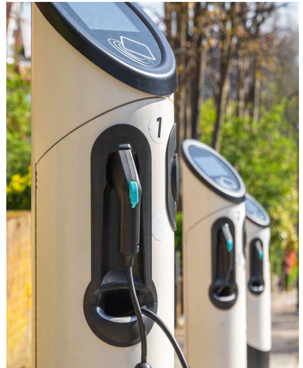
Figure 3 EV Charging Point
